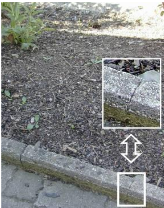
Fig. 2: Break in the kerb
