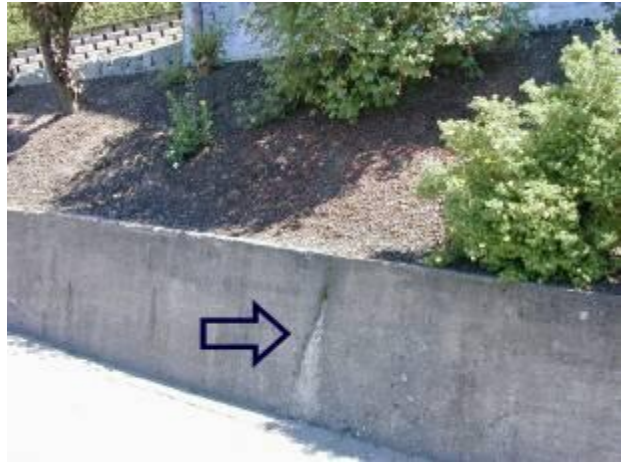
Fig. 1: Break in the wall
