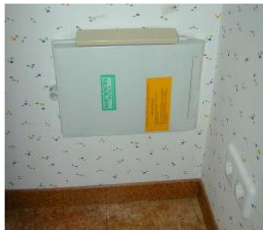
ELO-Rayex attached to the armour safety fuse box in the house
